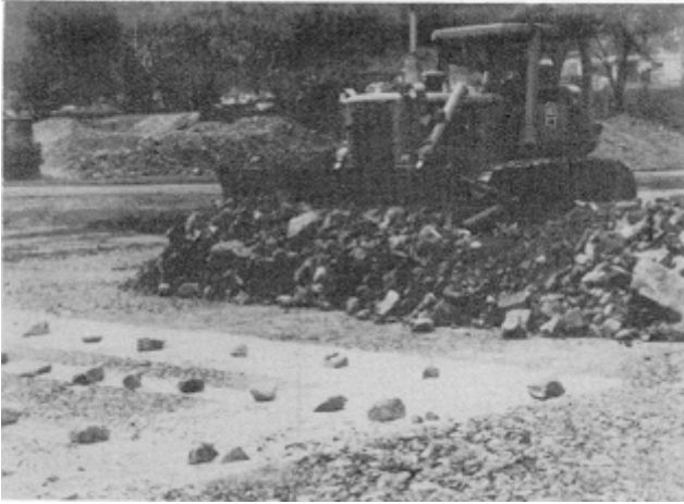
Figure 10-3. Placing a lift in the Cerrillos Dam test fill (Note the marking of the previous lift surface with plastic strips and lime)
