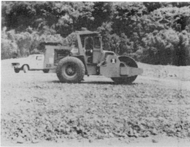
Figure 10-4. A 9.1 mg (10-ton) vibratory roller at work on the Cerrillos Dam test fill
